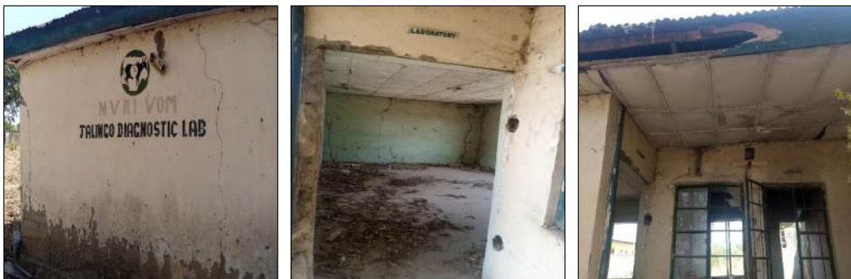
Figure 1: Dilapidated infrastructures in the NVRI Jalingo outstation.
